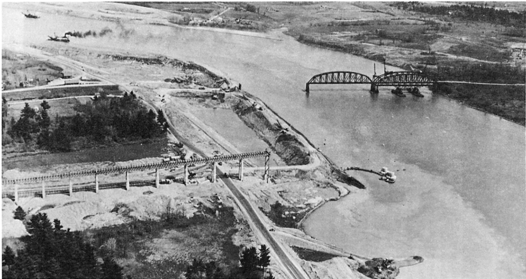
The partially removed Roosevelt Bridge, May 1958. Its north span rests on temporary piers. Also shown is the excavation on Cornwall Island and the partially built high-level bridge.
