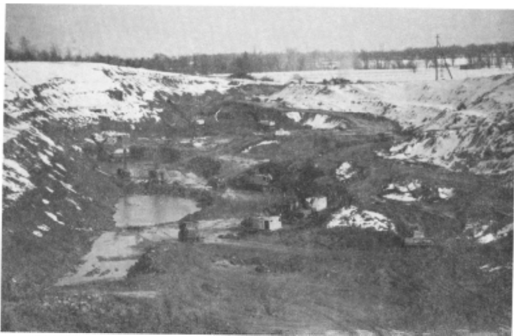
The drainage problem during construction, February 1956.
